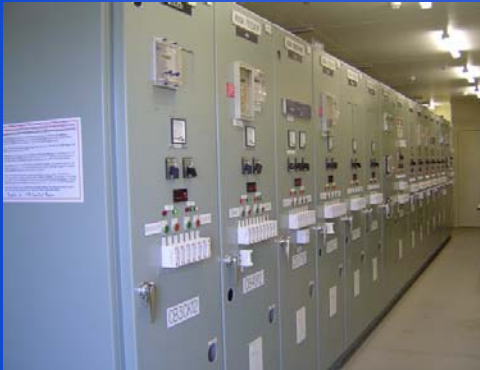
36kV Indoor Compact-GIS for EnergeX Ltd
