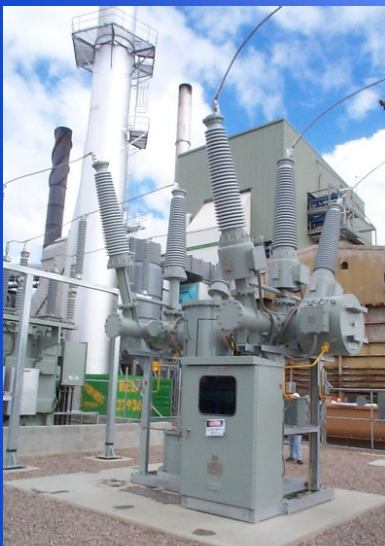
145kV Outdoor GIS for EnergeX Ltd
