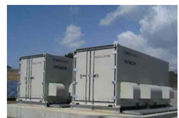
Example : Two PCSs installed in each container
