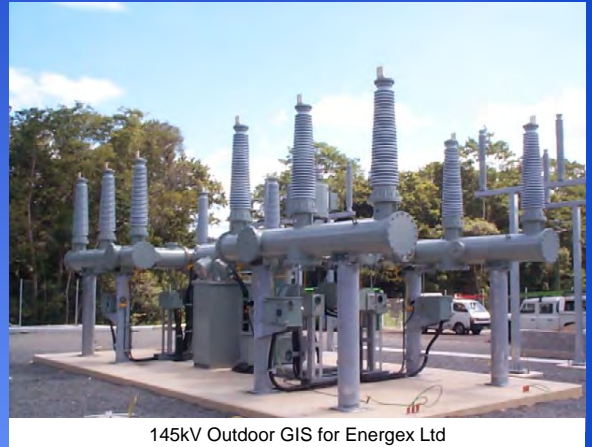
145kV Outdoor GIS for Energex Ltd
