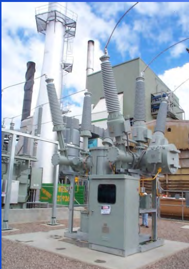
145kV Outdoor GIS for Energex Ltd
