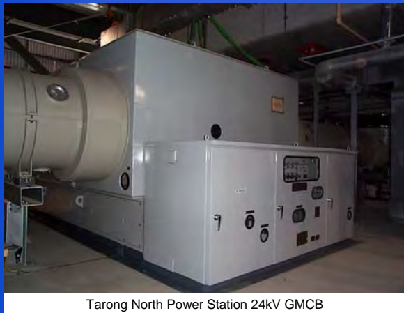
Tarong North Power Station 24kV GMCB
